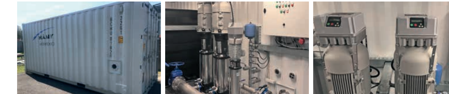
Water supply container
