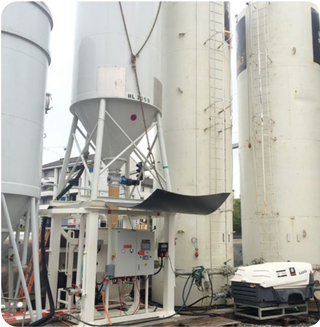
Häny HCM 800 mixing plant with storage silos
