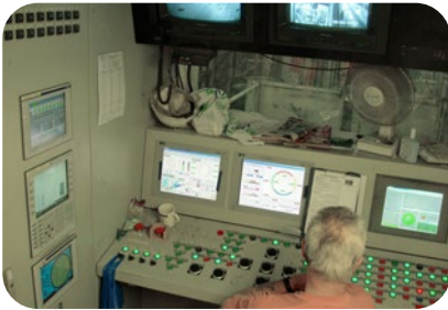
Kommandoraum TBM Control room of TBM
