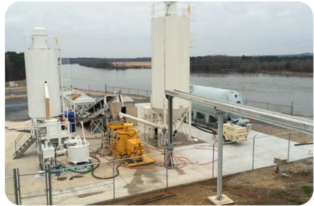
Häny mixing plant with the Lower Coosa River in the background
