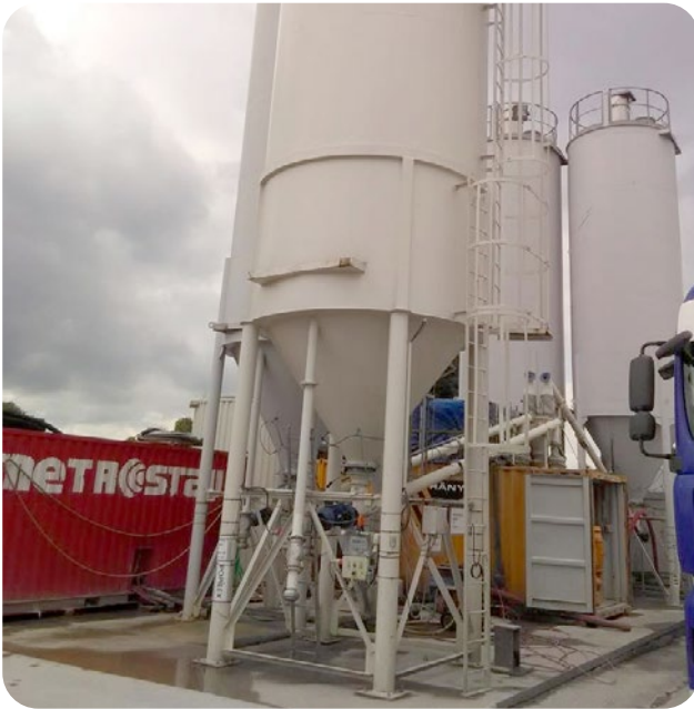
Häny MCM 5500 mixing plant, connected to 4 silos
